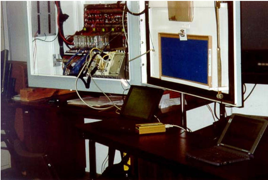
Figure 8 - Bench Testing the RACU with a NEMA Controller and Cabinet
