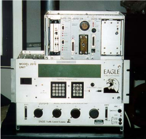
Figure 7 - RACU with a Model 2070 Traffic Controller
